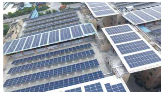
DONGGUAN 1MW PHOTOVOLTAIC PROJECT
