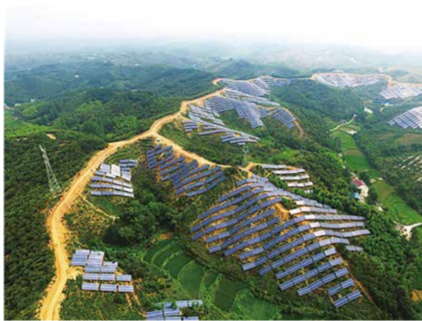
ANHUI 3.6MW POVERTY RELIEF GROUND PHOTOVOLTAIC POWER STATION
