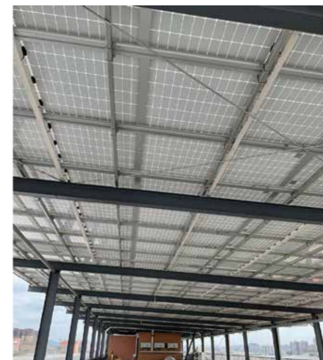
DONGGUAN 1MW PHOTOVOLTAIC PROJECT
